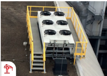
Walkway on a roof for servicing the A/C system
